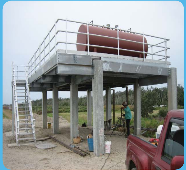
Construction progress of the North and South Florissant Drainage Pump Station Reconstruction Project in eastern St. Bernard Parish designed by HDCA
